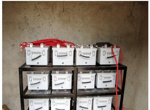
Twelve batteries hold electricity for the Bible Institute.
