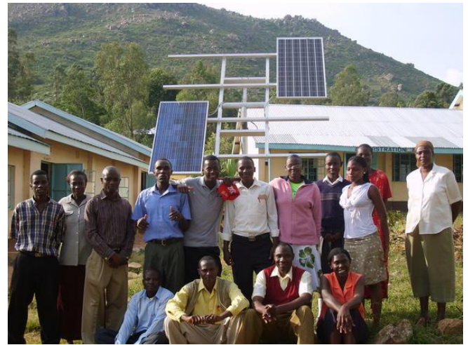
The emPower Plant™ at Mbaka Oromo Primary School, Kisumu Kenya, with space left for additional solar modules to be added later.
